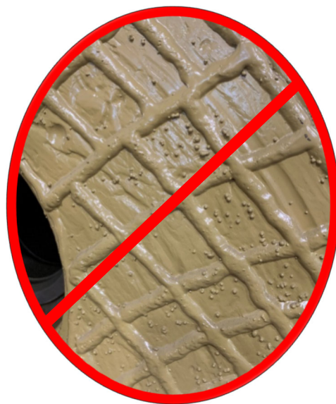
Figure 54 – Incorrect pattern on base plate
