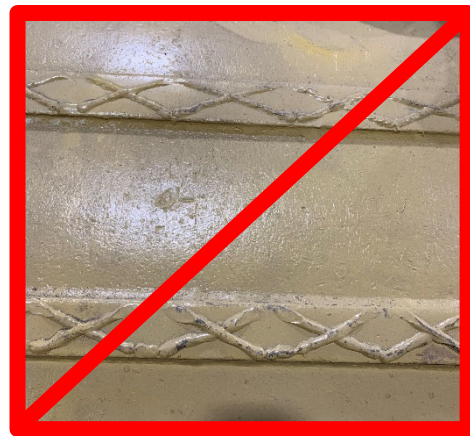
Figure 56 – Incorrect pattern on wear bars
